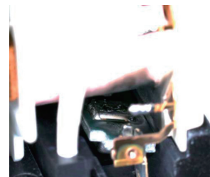
Burning of the CR element (circuit board)
