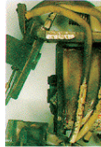
Burn damage due to overcurrent/overvoltage
